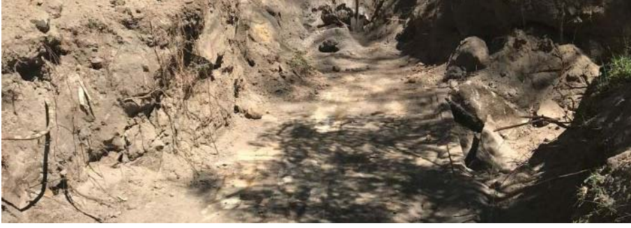
PHOTO: A buried concrete slab, which was not identified on military maps was uncovered. (Supplied: Charles Tennyson)
